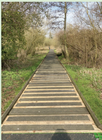
The foreground of this photo shows 16 new boards – cost £240
